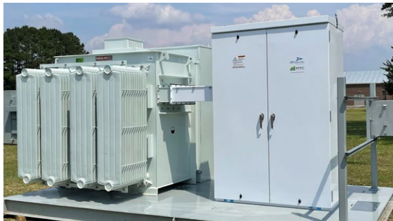
PV UNIT SUBSTATION
