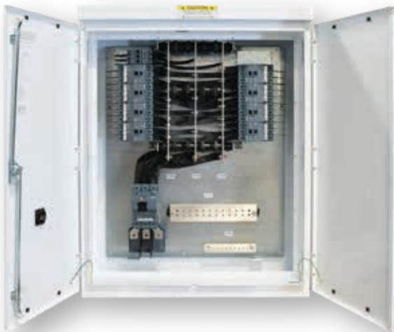
Pictured above: UL / NEMA 3R, 600A AC BESS MLO distribution panel, Internal view, No deadfront.
