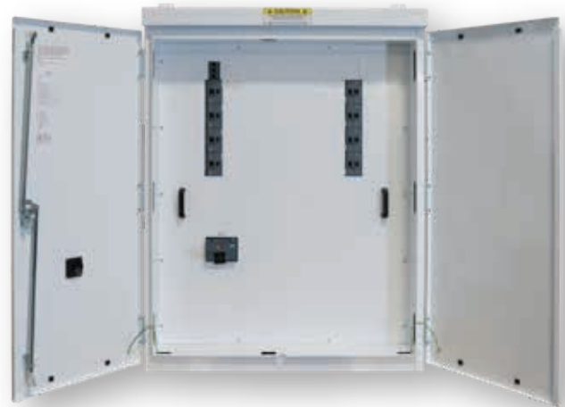
Pictured above: UL / NEMA 3R, 600A AC BESS distribution panel, external view
