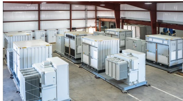
CENTRAL INVERTER STATION
